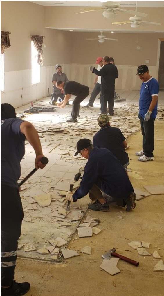
Camino a Cristo church members help remodel their new facility purchased this year. Photo: Noreen Vargas
